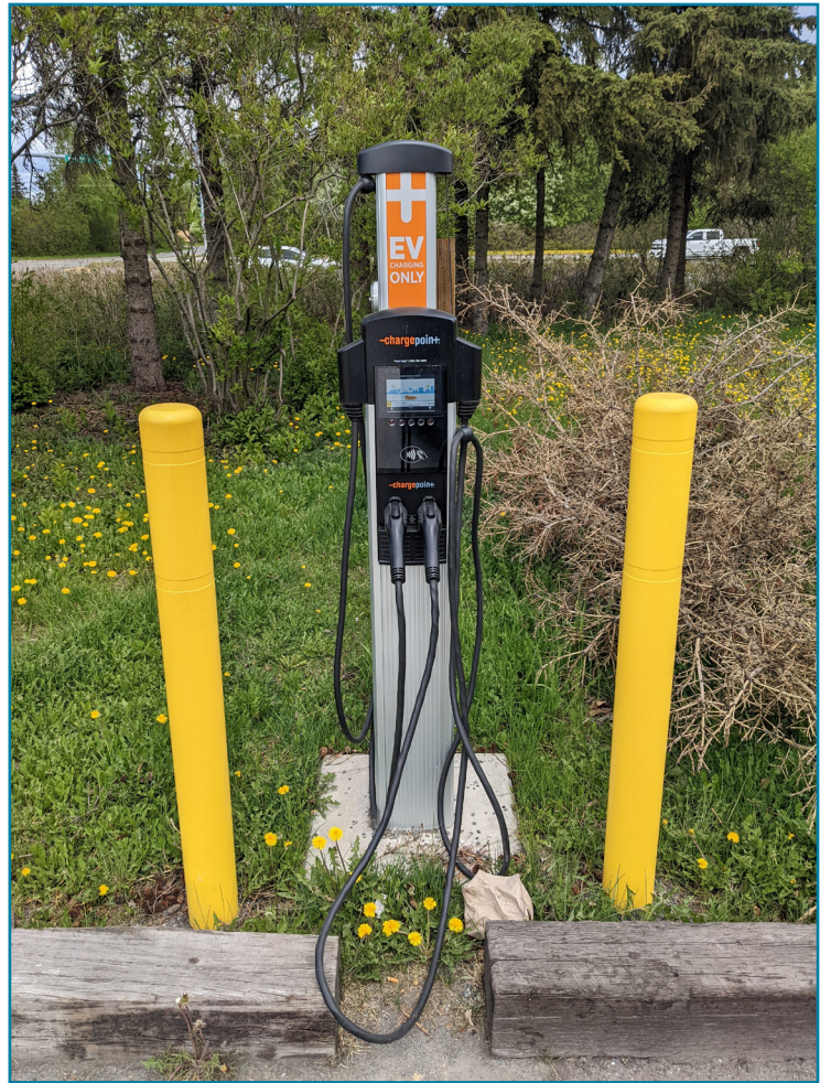
Charging station on Northern Lights Blvd in Anchorage, Photo courtesy of AEA
