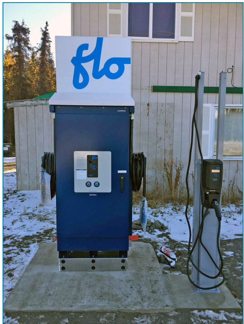
AEA-funded EV charging stations in Cantwell Photo courtesy of AEA
